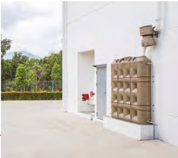
Rainwater Harvesting Tank at i-Park's Factories
